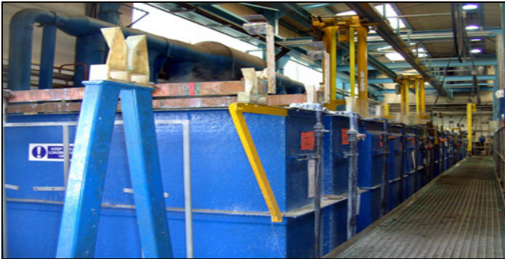
Apticote 300 Automated Anodising Line
